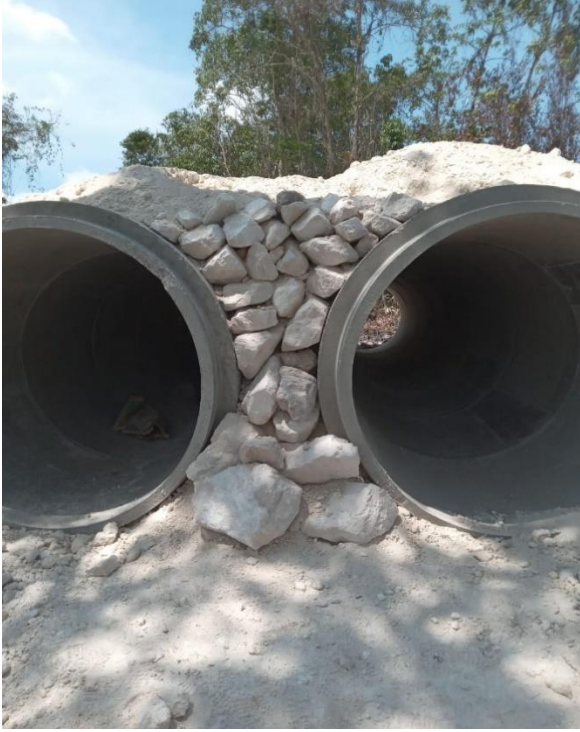
Double concrete culverts with stone pitching end treatment - Yo Creek Sugar Road
